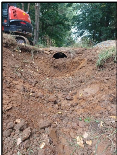
Above: The ditch to the east of Scaldwell stream after deepening. The culvert pipe is relatively small and mostly blocked with silt.
