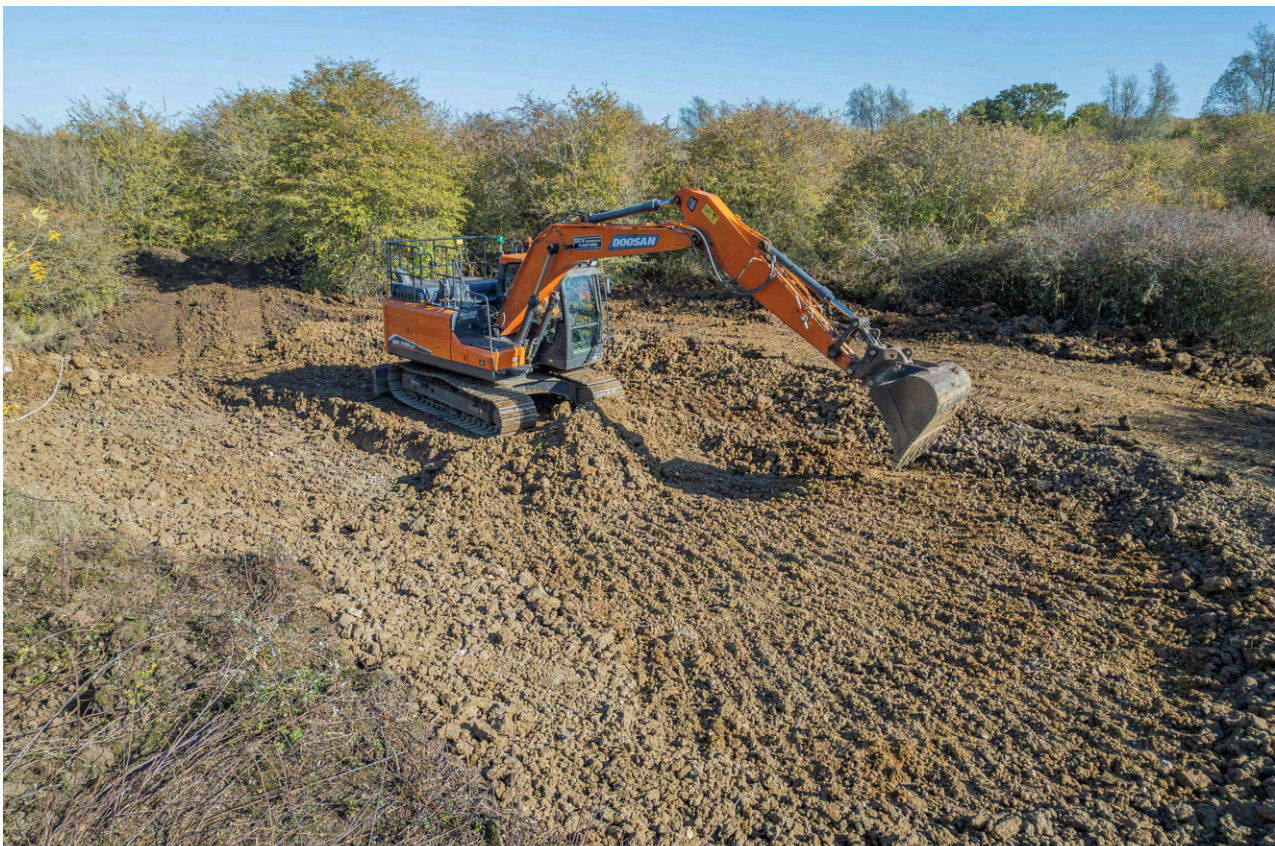
Figure 6: Work commenced on the construction of six new ponds at Strawberry Hill in October 2025 (Photo: H. Wilkinson)
